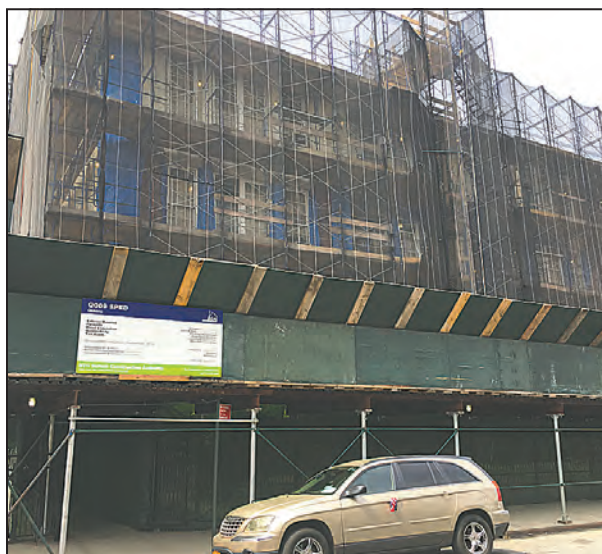
District 75 school PS 9 in Maspeth is a dark, dusty and dilapidated building in which students with special needs should not be learning, according to Councilman Bob Holden.
